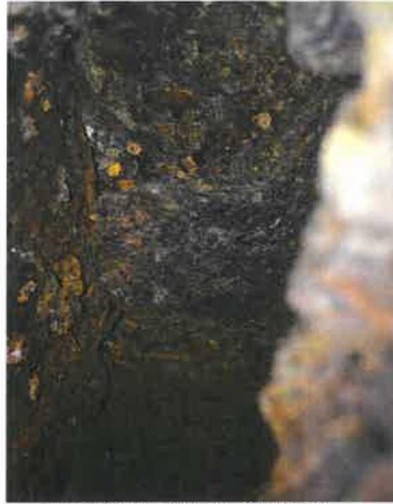
(Photo #2) East Stringer: Rust on Interior of Bottom Chord
