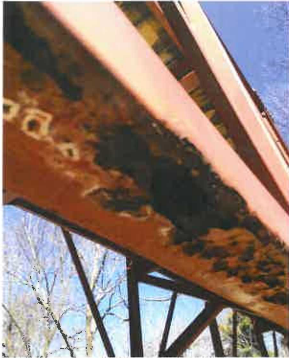
(Photo #1) East Stringer: Rust on Underside of Bottom Chord
