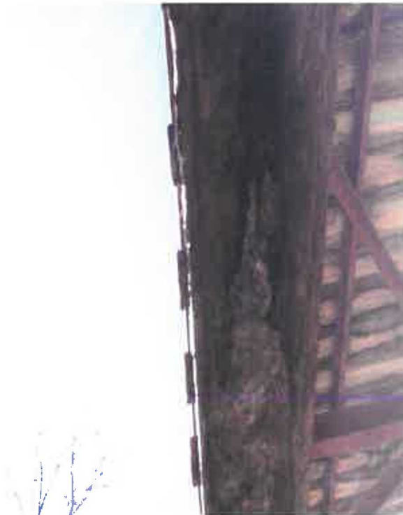
(Photo #7) West Stringer: Rust at Splice Connection
