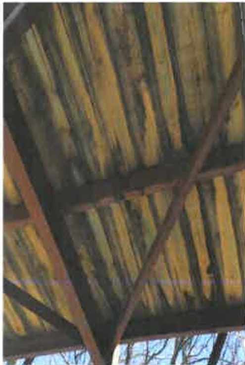
(Photo #8) Rust at Underside of Plank Support Steel
