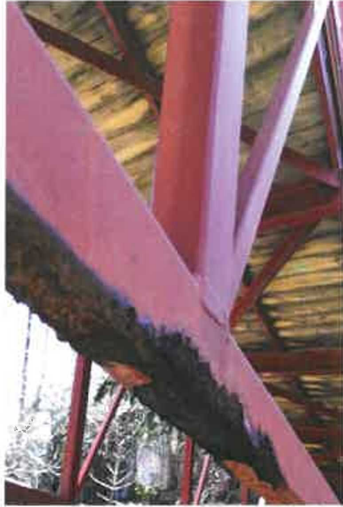
(Photo #6) West Stringer: Rust on Bottom Chord
