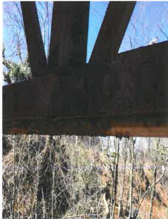
(Photo #4) East Stringer: Rust at Splice Connection
