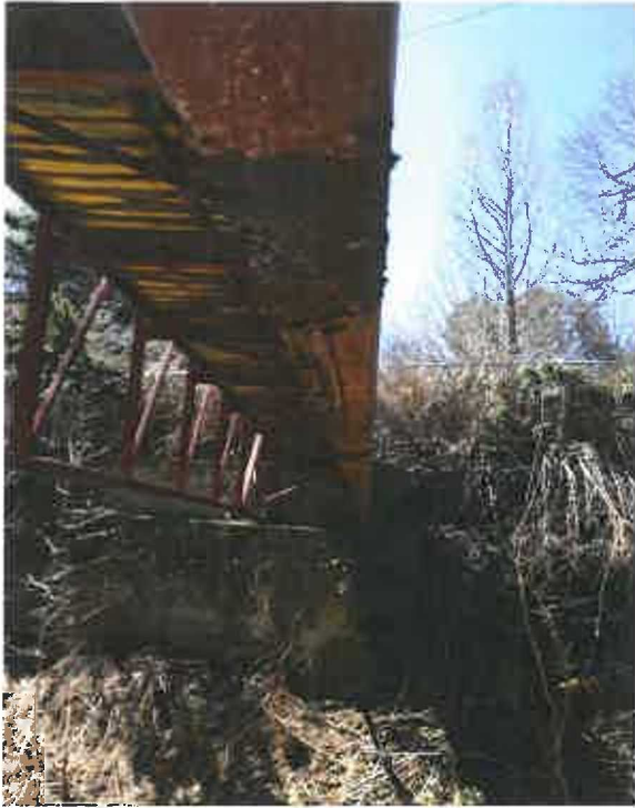
(Photo #5) West Stringer: Rust on Bottom Chord
