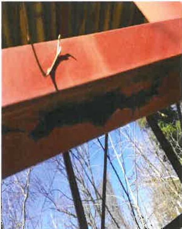
(Photo #3) East Stringer: Rust on Underside of Bottom Chord
